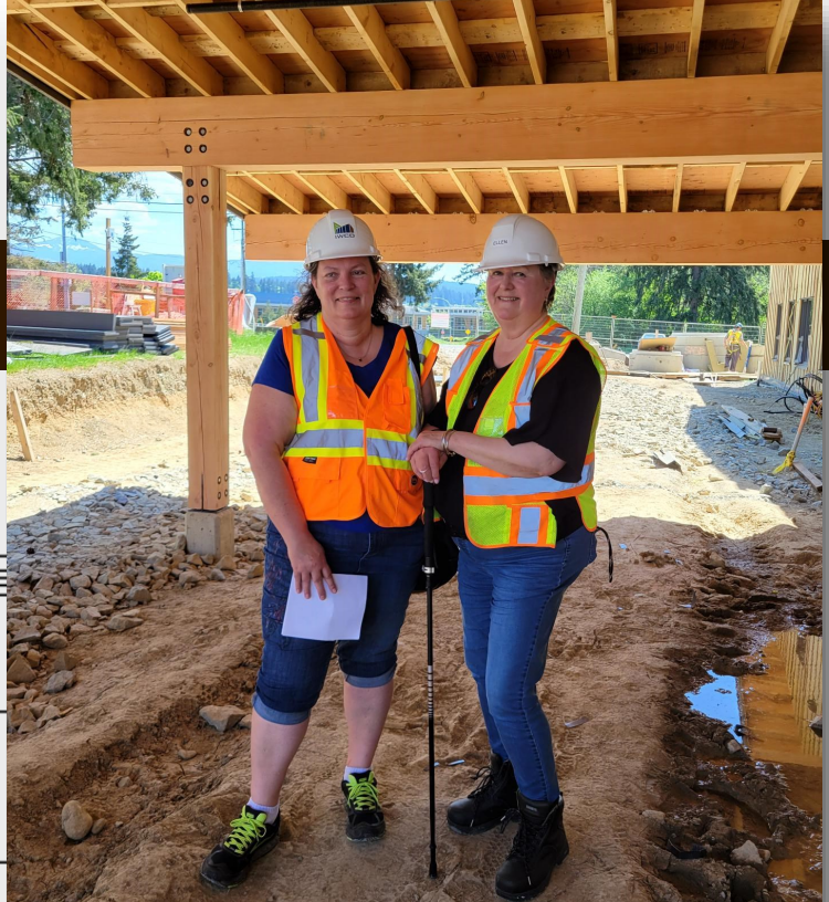
Cindy Blake and Ellen Froid at the construction site of BC Housing and Sage Haven's Second Stage Housing Project.
